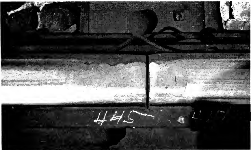
Fig. 7—Photograph of joint 2 showing a transverse crack in weld metal of west rail.
